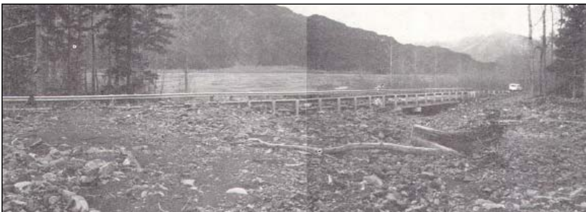
Figure 26: Cobble and gravel deposits at Bridge 1389, Mile Post 4.7 Exit Glacier Road. View downstream on October 13, 1986.
