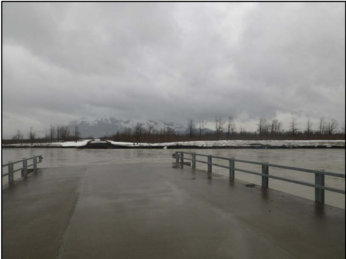
Figure 1 – Road breach looking east June 4, 2013
