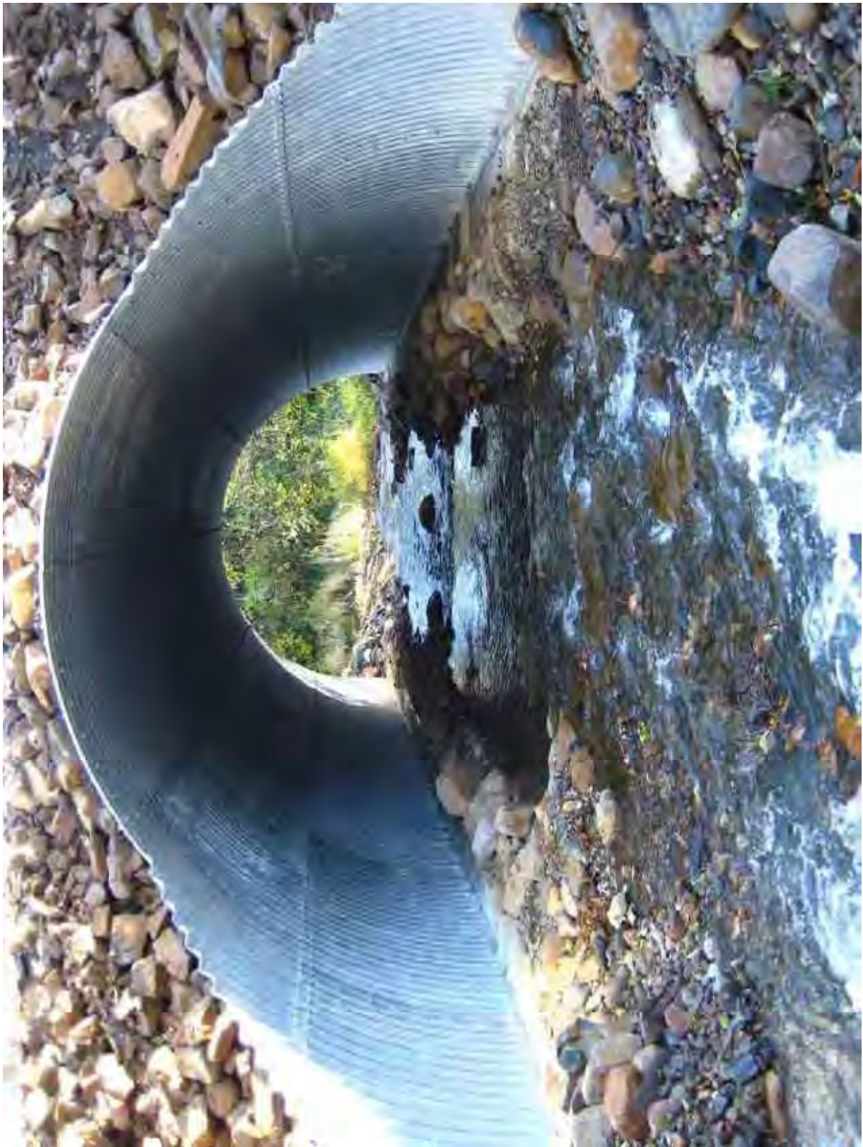
Figure 4. This arched-culvert example shows the diverse water depths and velocities, hiding and resting areas, and moist-edge habitats that support aquatic species movement.
