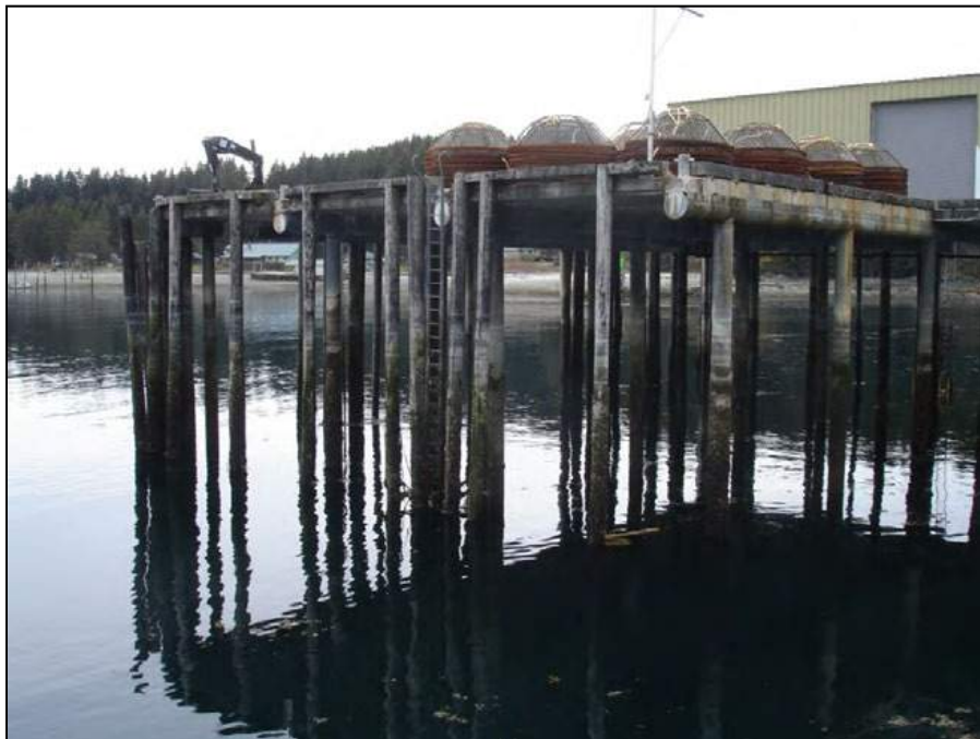
Figure 16: The city dock seen from the ferry dock. While the piles appear to be in good condition, the deck has some severe edge damage and is probably incapable of handling heavy cargo transfer.
