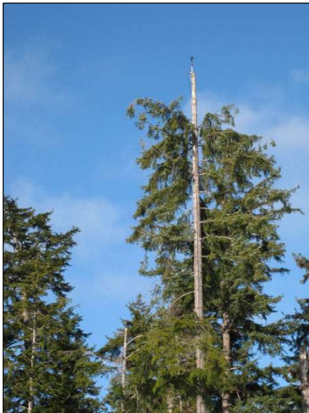
Example of wind meter after installation.
