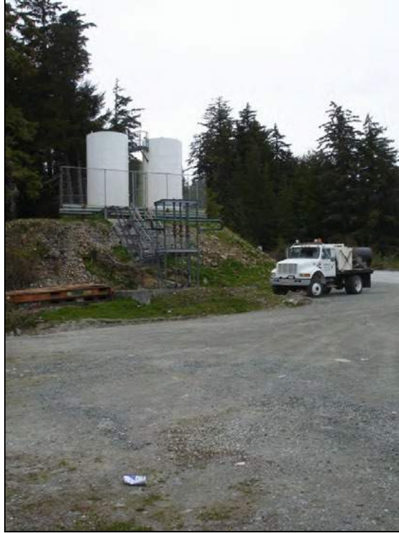
Figure 9: Fuel storage tanks at Killisnoo Harbor. Maximum storage capacity is 36,000 gallons.
