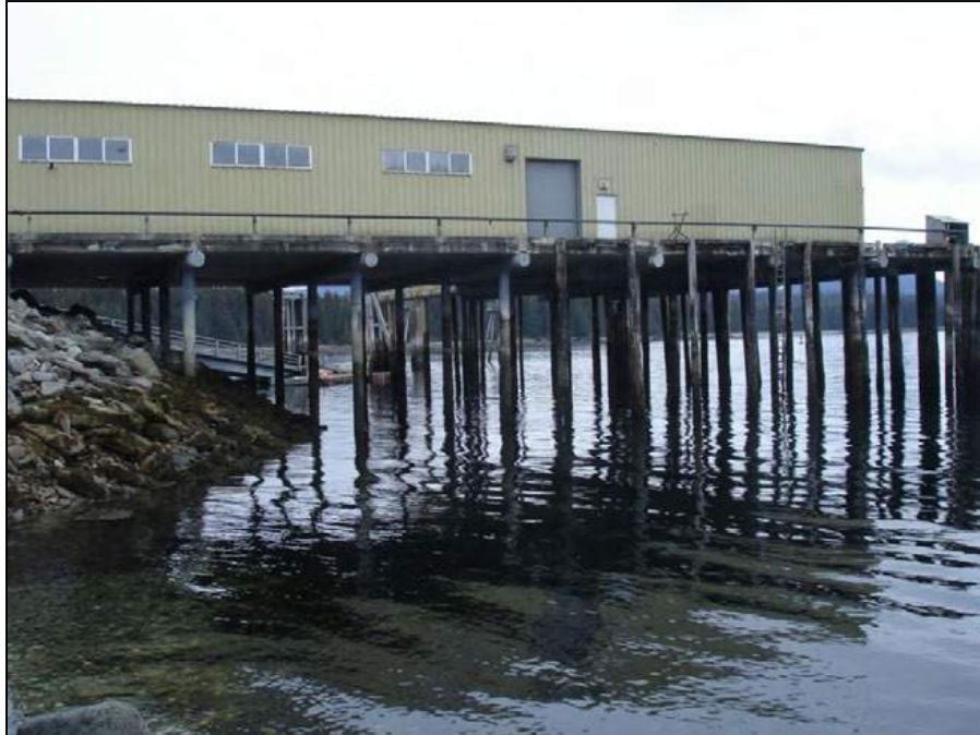
Figure 15: West face of the city dock. Some of the fender piles are damaged.
