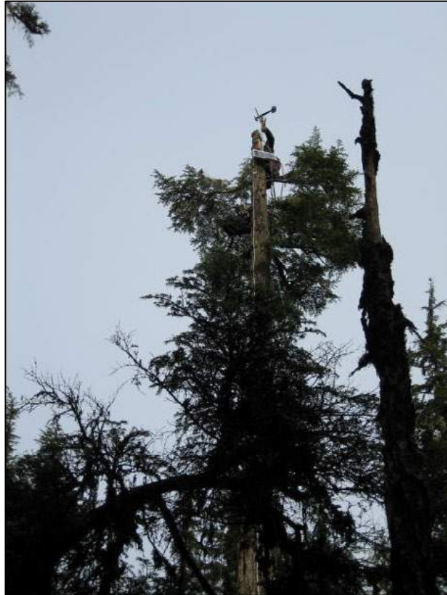
Installation of the equipment at near ADOT&PF's Master Plan preferred airport site.
