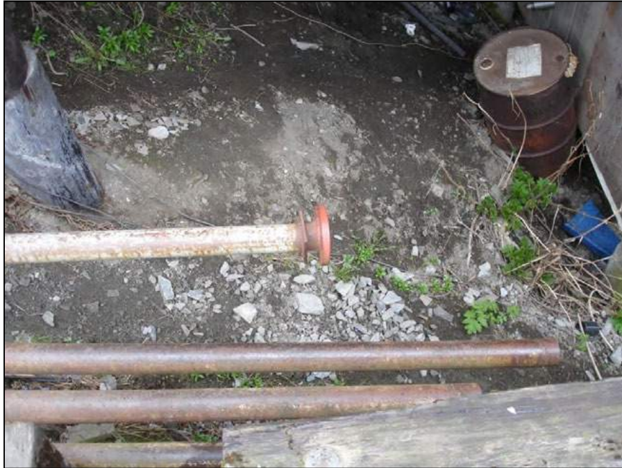
Figure 6: De-commissioned fuel piping under the Chatham Strait Dock.
