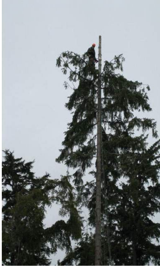
Preparing the tree for installation of the equipment at the water tower site.
