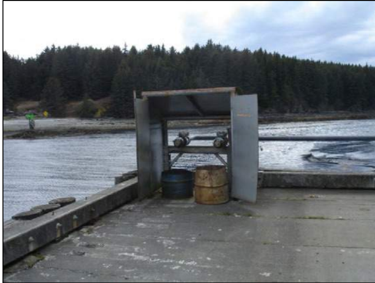
Figure 7: Fuel headers on the southwest corner of the city dock.
