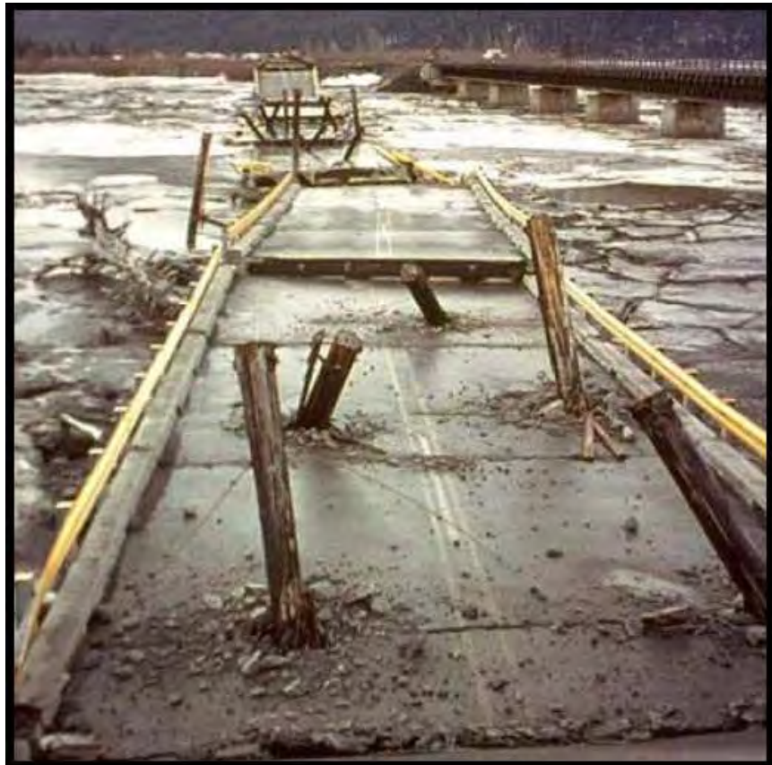
Photograph 2: Example of Bridge Damage from Earthquake
