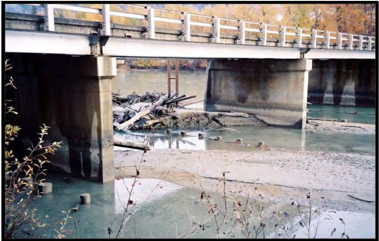
Photograph 4: Logjam Underneath Bridge
