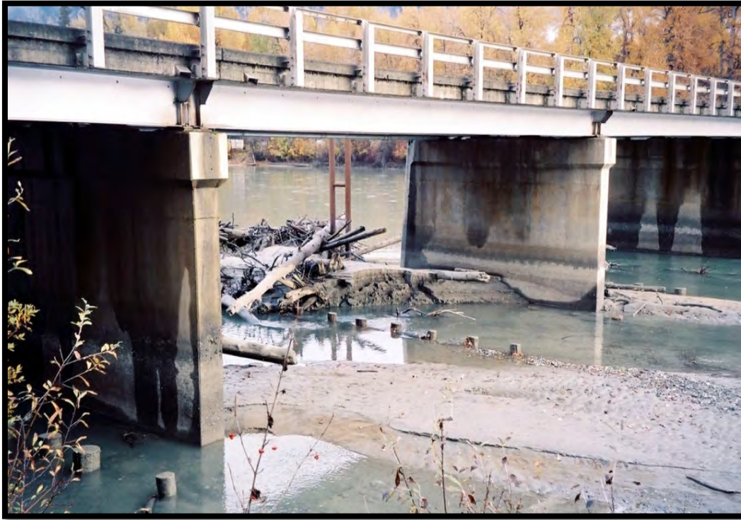
Photograph 4.12-1: Logjam Underneath Bridge
