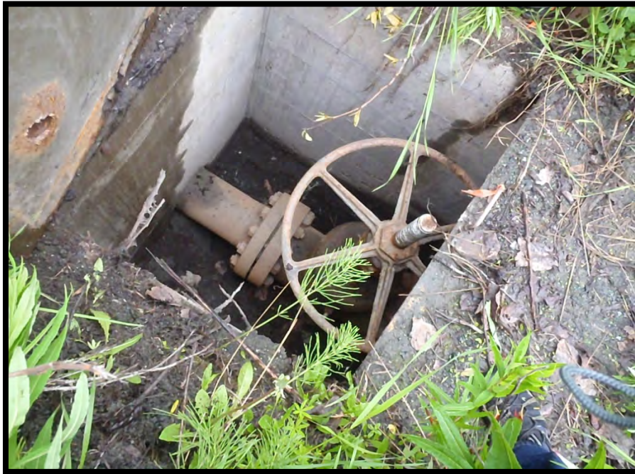
Photograph 4.10-1: Haines-Fairbanks Pipeline Gate Valve 4
