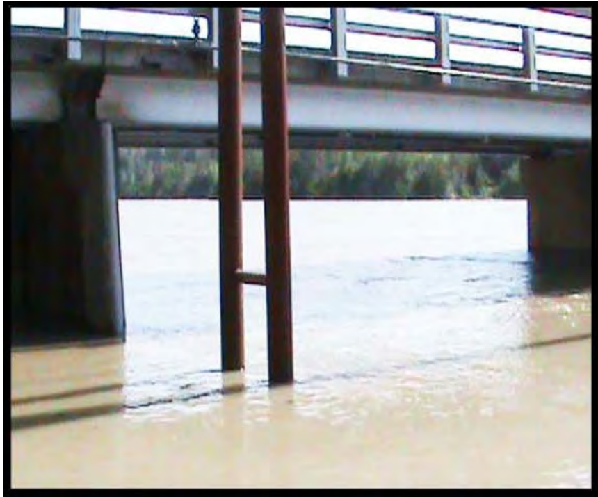
Photograph 3: Bridge Low Clearance
