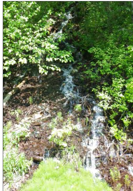
Figure 2.—Barrier falls on ditch at wpt 46.
