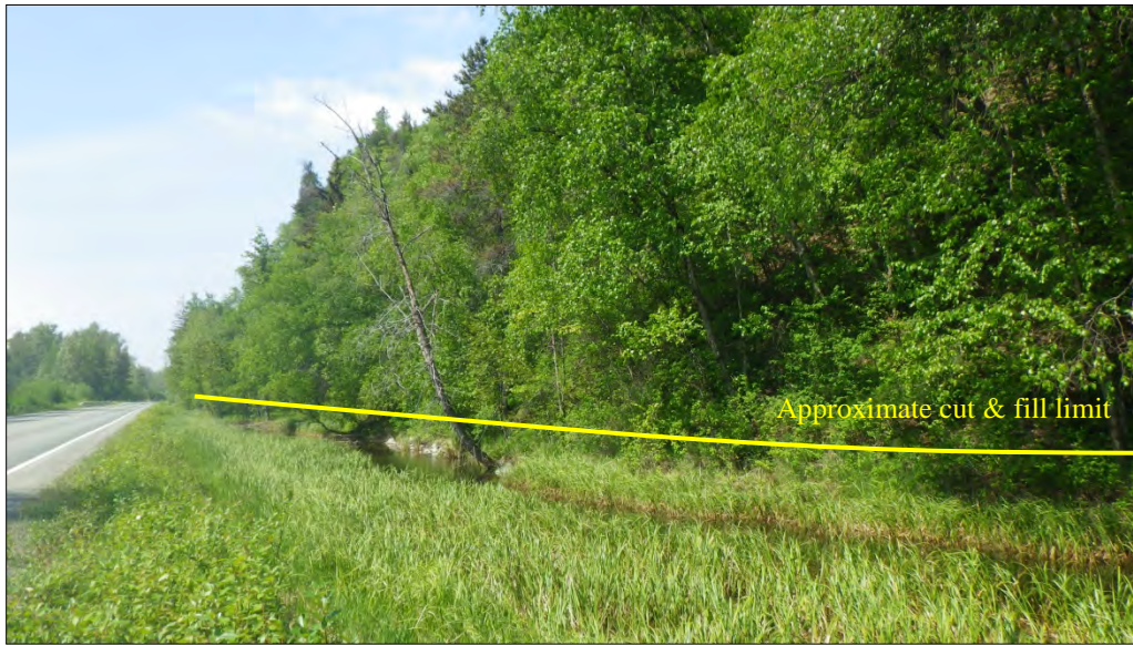
Figure 27.–MP15.0 ditch drainage falls adjacent to HH.
