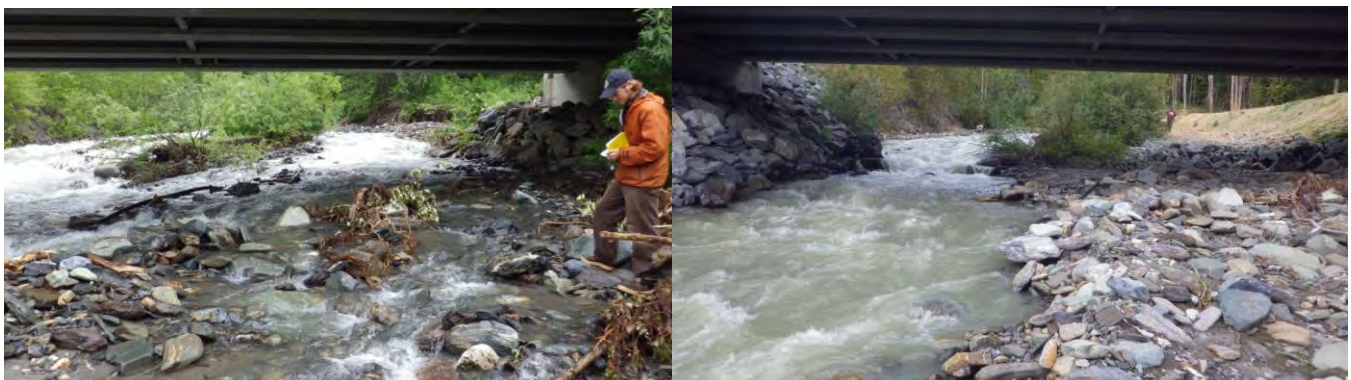
Figures 9 & 10. Left: Looking upstream from below Little Boulder Creek bridge before the launch apron raised the elevation in the overflow channel on river left (June 27, 2012). Right: Same view following embankment repairs with dry, elevated overflow channel (September 4, 2013).
