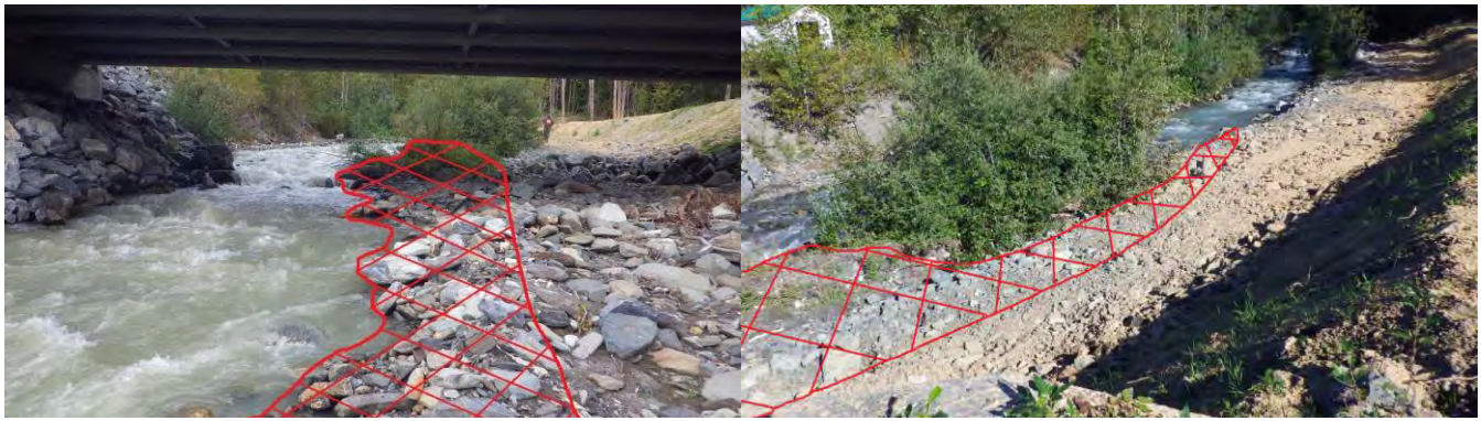
Figures 11 & 12. Left: Looking upstream from beneath the bridge at constricted section with recommended fill removal outline in red. Right: Looking upstream from the bridge with approximate recommended fill removal outline in red.
