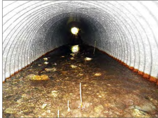
Figure 35.—Stream No. 115-32-10250-2070 culvert outlet, looking upstream. Photo courtesy of Matt Eisenman and Jim Latham, ADF&G Division of Sport Fish.
