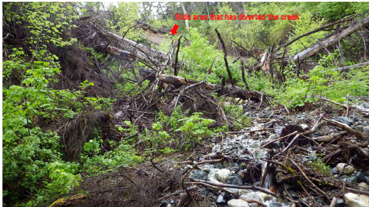
Figure 4. Looking upstream above the highway at stream no. 115-32-10250-2016-3020 headwaters and a landslide. The arrow shows where the slide occurred that diverted the creek.
