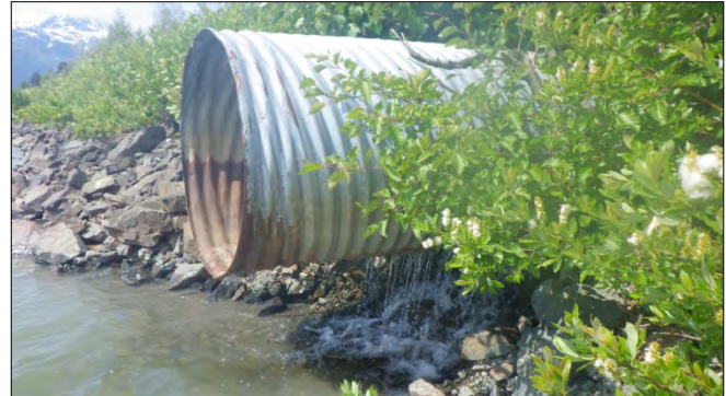
Figure 16.–Stream No. 115-32-10250-2024 HH culvert (FP12) outlet, perched and corroded.
