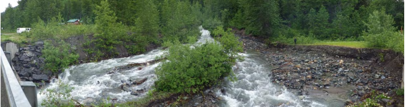
Figure 4. Looking upstream from the bridge with recent erosion visible on the right side. High flows directed an overflow channel toward the eastern abutment of the bridge (June 27, 2012).
