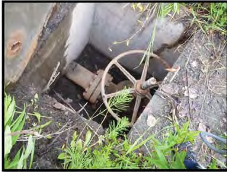
Photograph 4.10-1: Haines-Fairbanks Pipeline Gate Valve 4
