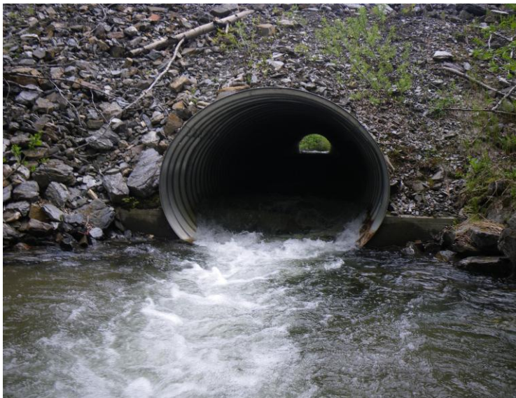
Figure 15.–Culvert CV-13 outlet with baffles.
