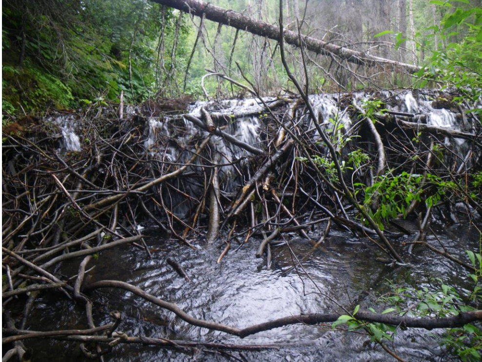
Figure 11.—Beaver dam downstream of culvert CV-11 and CV-12.
