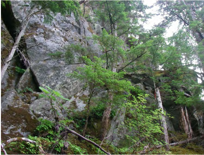
RF27. View south/down alignment at rockfall hazard.
