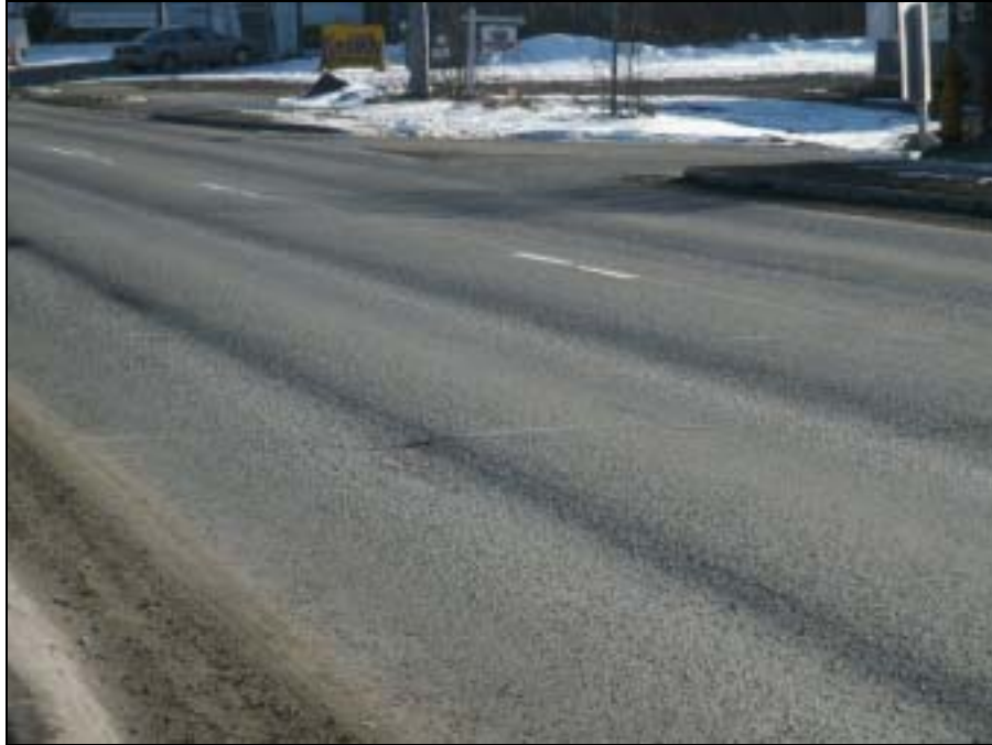
Figure 6.1. Pavement rutting in Anchorage, Alaska (Photo: Stan Porhola)
