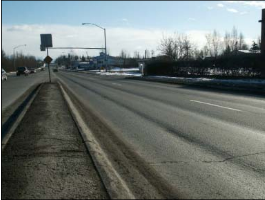
Figure 1.1. Pavement Rutting on Lake Otis Parkway in Anchorage, Alaska
